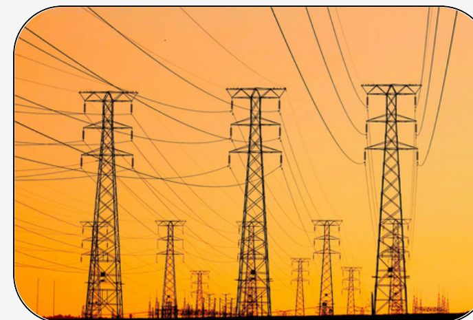
Wire and Transmission
